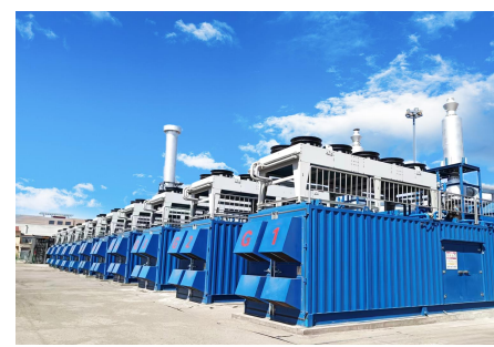
LANDFILL GAS POWER GENERATION PROJECT
